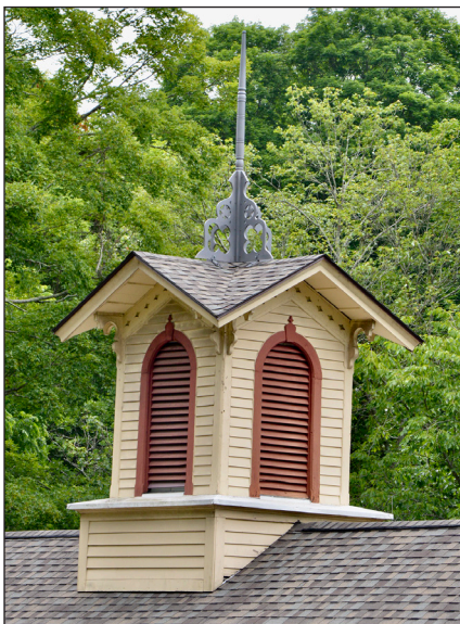
Following the installation of the new roof shingles and gutters at the museum, member Art Christianson crafted a handsome spire to top the cupola, replacing the historic one that fell a few years ago.
