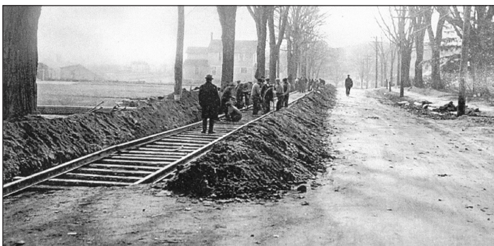
Tracks being laid in 1913 along Middlesex Turnpike near St. Joseph Church in preparation for the extension of trolley service to Chester in early 1914. (Hugh Spencer photo from Society archives)
